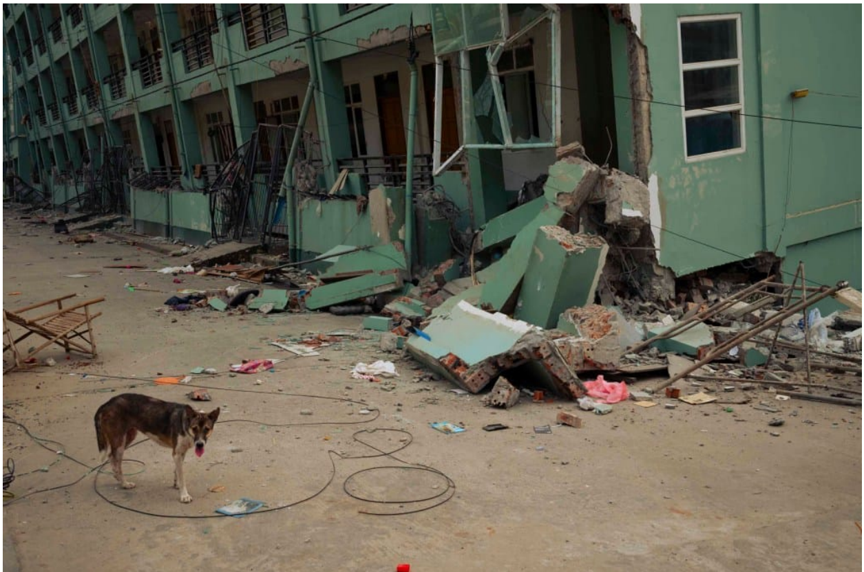
An apartment building destroyed by the earthquake. Photo: Patrick Chengzhi Wang
