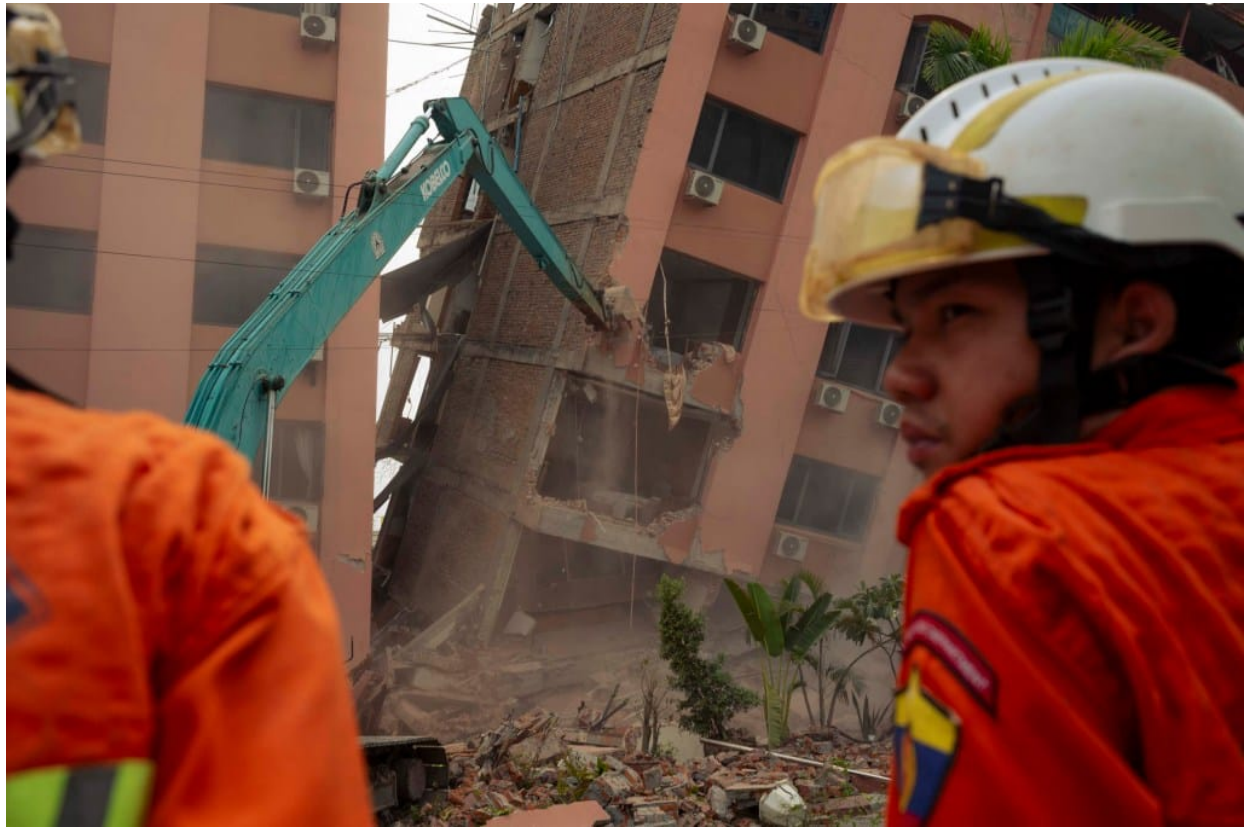
Earthquake damage at the Great Wall Hotel. Total casualties unknown. Photo: Patrick Chengzhi Wang
