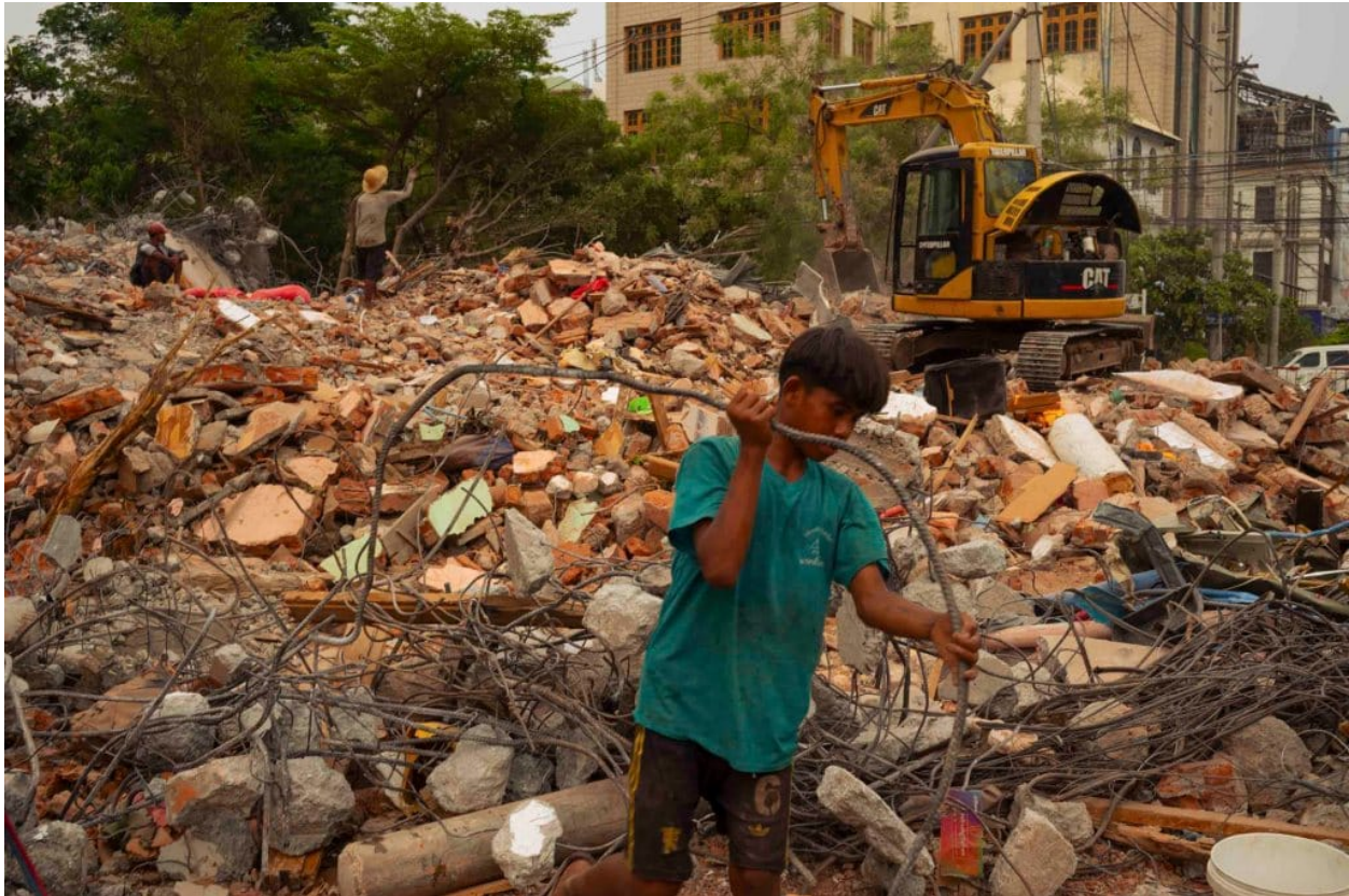
A teenager carries mangled rebar as he walks out from the collapsed ruins. Photo: Patrick Chengzhi Wang
