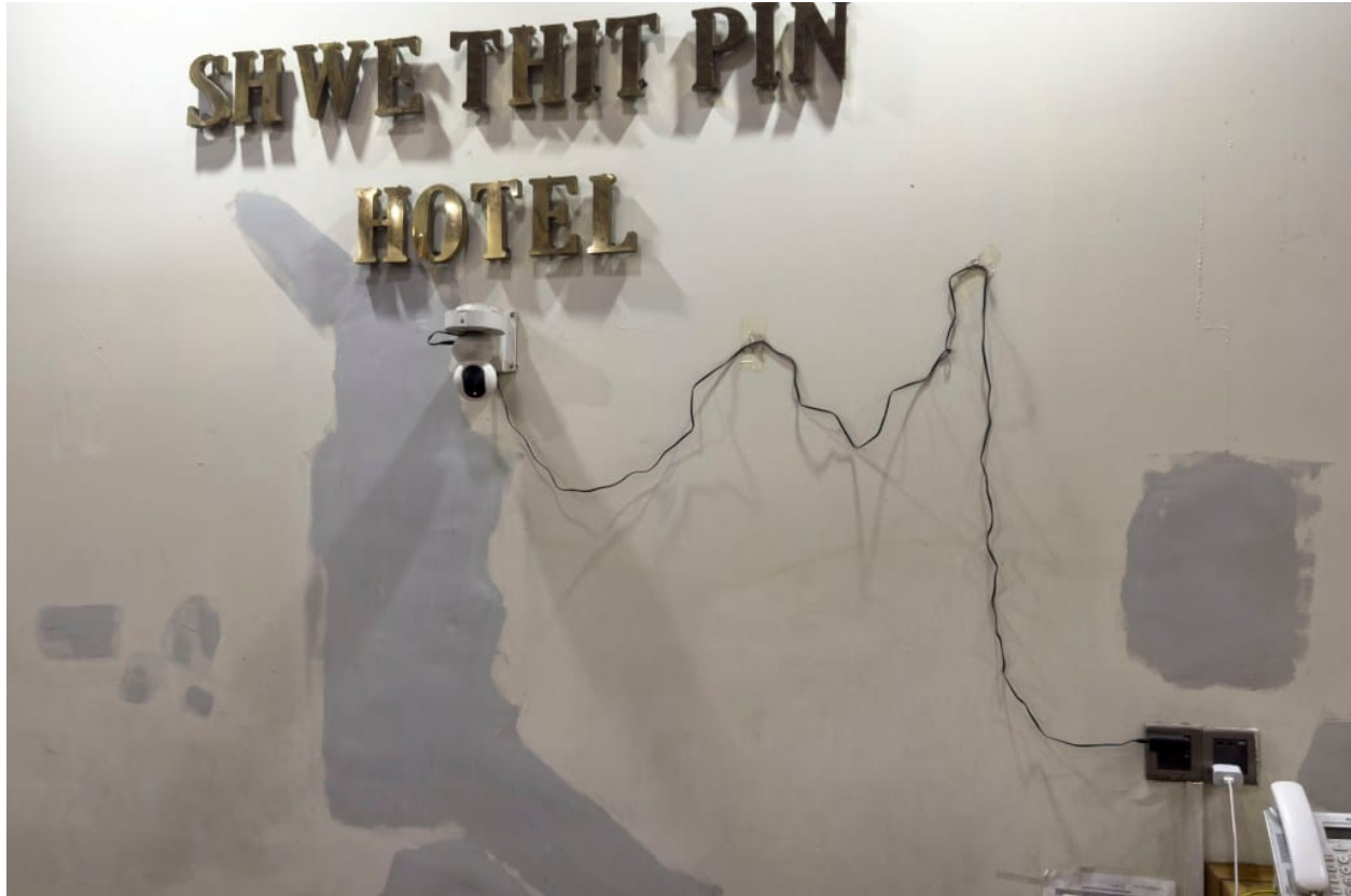
The hotel walls are riddled with cracks. Photo: Patrick Chengzhi Wang
