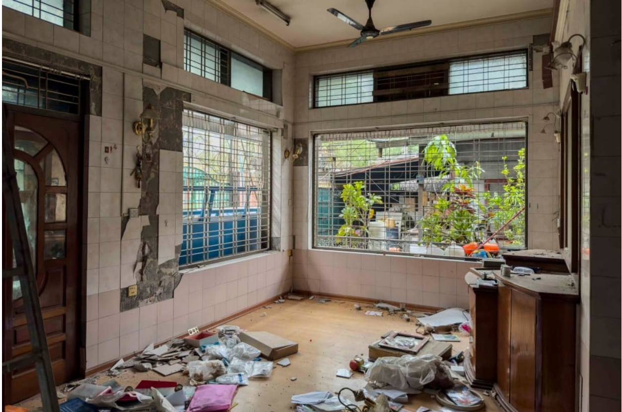
The damaged house of Jonn’s family. Photo: Patrick Chengzhi Wang
