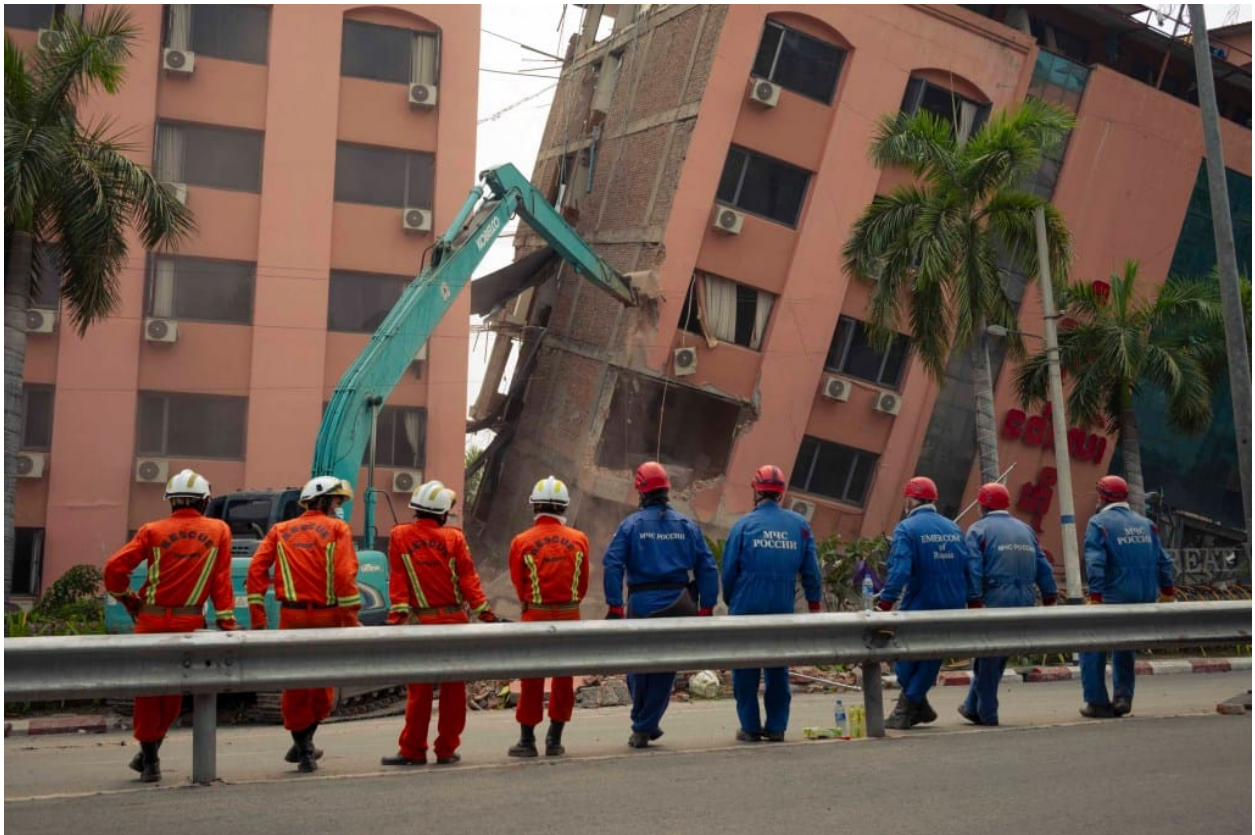
Demolition of the structurally unsound Great Wall Hotel. Nearby, Myanmar (orange) and Russian (blue) rescue teams take a break. Photo: Patrick Chengzhi Wang
